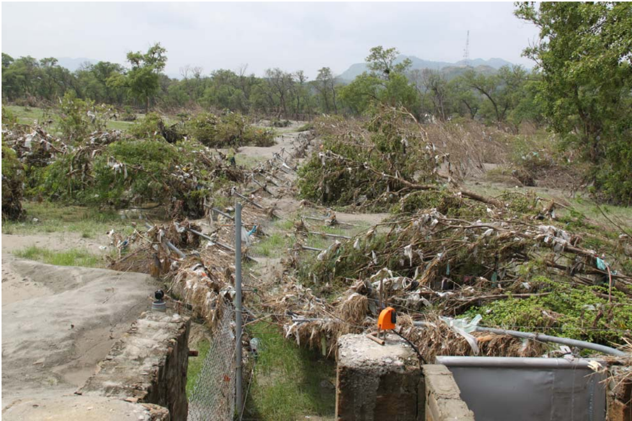
Figure 10: Glimpse of damage in Kund Park/photo Ayaz Khan, PWP
